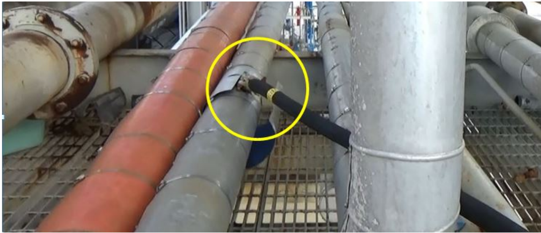
Figure 14. Hot water hose positioned on the liquid methyl mercaptan feed piping to flow hot water between the piping and the insulation in an effort to heat the piping and dissociate the solid hydrate that formed after water inadvertently entered the mercaptan storage tank.
