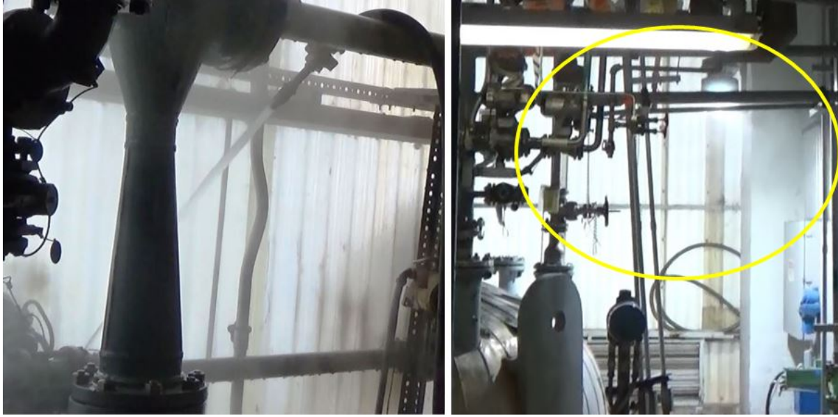
Figure 24. Ineffective ventilation on the second floor of the manufacturing building. These photos document an operational activity taking place on January 9, 2015. Operations had directed a hot water hose on a flow meter on the north east side of the second floor as seen in the photo on the left. The photo on the right shows the steam nearly motionless (yellow circle) on the south east side of the building also on the second floor. Although the wet end fan was running at the time, an open door (Figure 25) provided a less restrictive path for air to enter the building and thus very little dilution air ventilation was taking place to sweep potentially hazardous gases out of the south east corner of the room. Note – these photos are snippets from a video recording. The video recording does a much better job of demonstrating the poor ventilation within the yellow circle.
