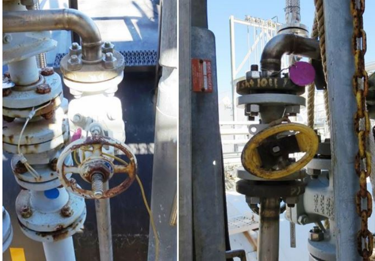
Figure 17. The fully open valve (left photo) and the cracked open valve (right photo) between the methyl mercaptan feed line and the waste gas vent header. These post-incident photos show the valve positions at the time of the incident.
