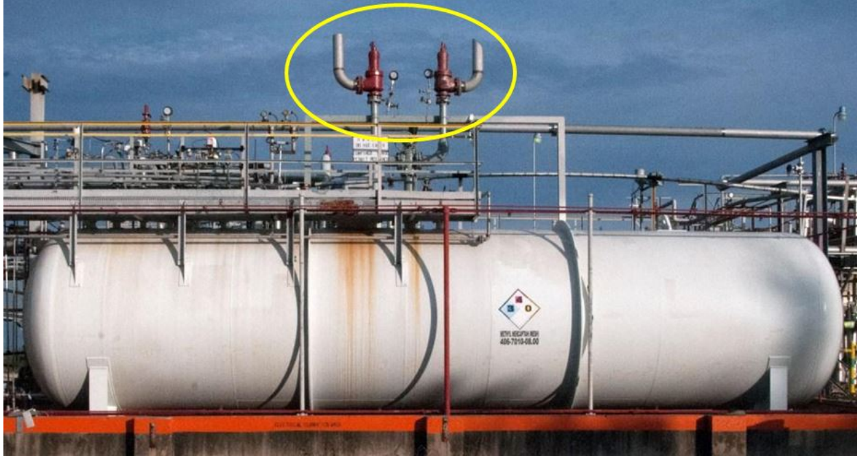
Figure 26. Methyl mercaptan storage tank showing atmospheric relief valves (yellow circle). At present, the storage tank is not insulated and there does not appear to be any mitigation to prevent off-site ERPG-3 concentrations as required by American Petroleum Institute and DuPont standards.
