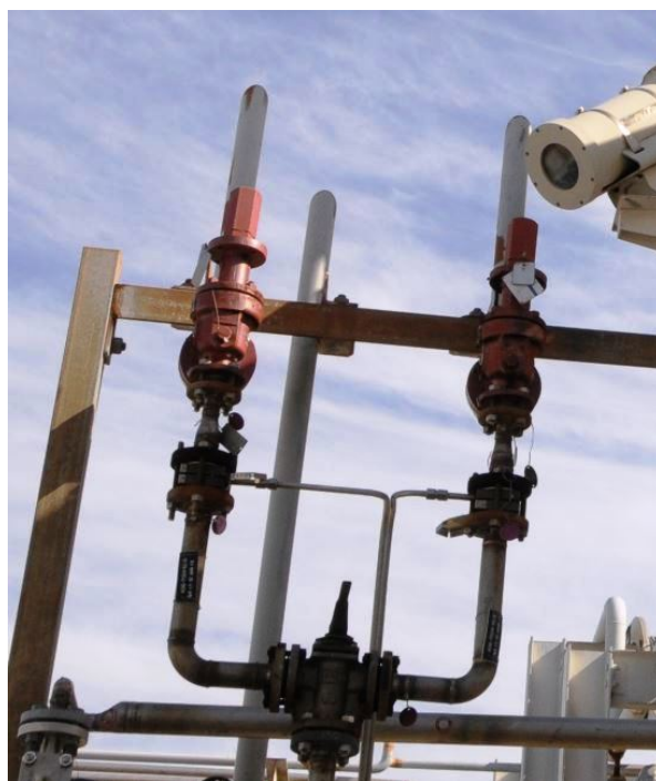
Figure 30. This photograph shows the nitrogen relief valves at one of the two methyl mercaptan railcar unloading stations. The nitrogen relief systems for each of the two railcar unloading stations are nearly identical. DuPont PHAs and relief valve design documents never considered the possibility of the methyl mercaptan storage tank pumps being lined up to these relief valves – as it was at the time of the incident. As a result, liquid methyl mercaptan was discharged from a system designed for nitrogen vapor.
