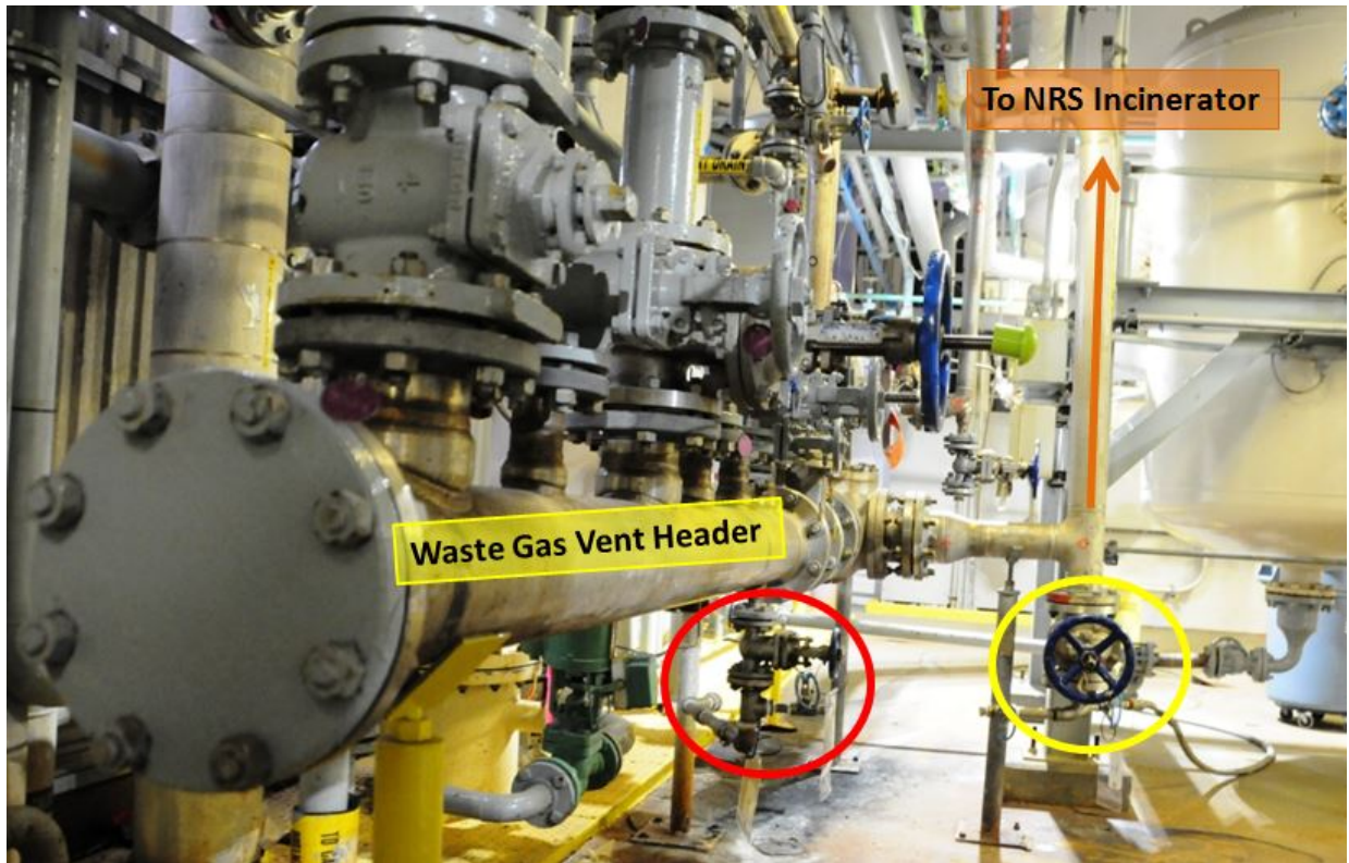
Figure 10. Waste gas vent header piping on the third floor of the manufacturing building. This portion, where several waste gas sources come together, is referred to as the waste gas vent header. Waste gas from this portion of the vent header travels up to reach the NRS Incinerator, a piping configuration that creates a low spot where liquid accumulates. To remove the liquid during waste gas vent header piping high pressure events, operators were instructed to open valves (yellow circle) and drain the system through a hose routed to a floor drain located near a safety shower. The floor drain is connected an open trench-type sump on the first floor. At the time of the incident, a second set of drain valves (red circle) were also opened directly to the floor inside the manufacturing building. This photo was taken while facing south. See Figure 11 for a view of the equipment while facing north.
