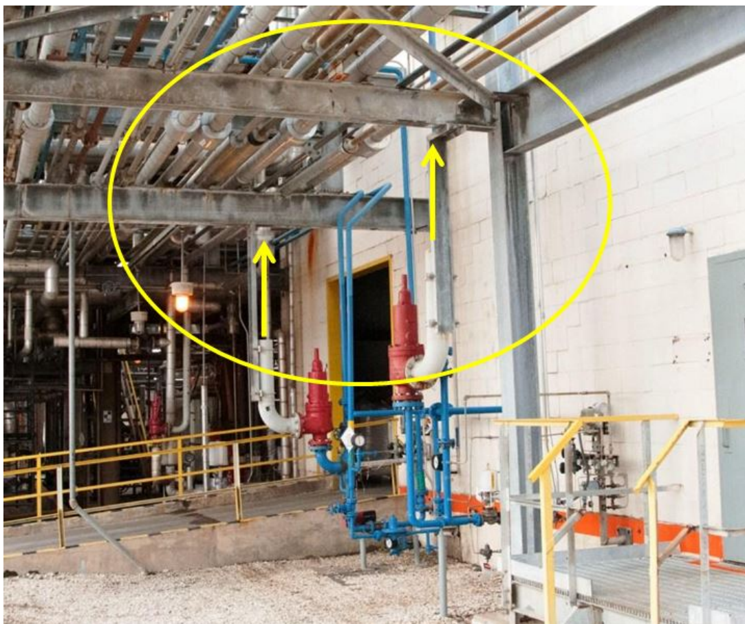
Figure 27. Nitrogen relief valves near south entrance of the manufacturing building. Dispersion from these atmospheric nitrogen relief valves is obstructed by an overhead pipe rack. This obstruction could result in a dangerous atmosphere to workers as they access or exit from the manufacturing building.
