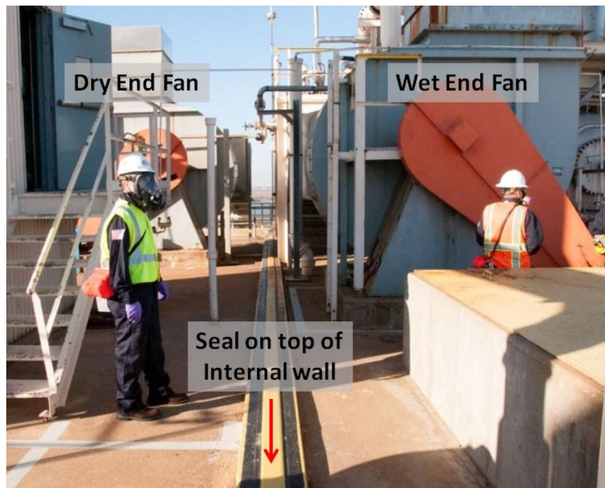
Figure 4. Roof of the manufacturing building showing the dry end fan (left), wet end fan (right), and location of the internal wall (middle) that separates each side within the building.
