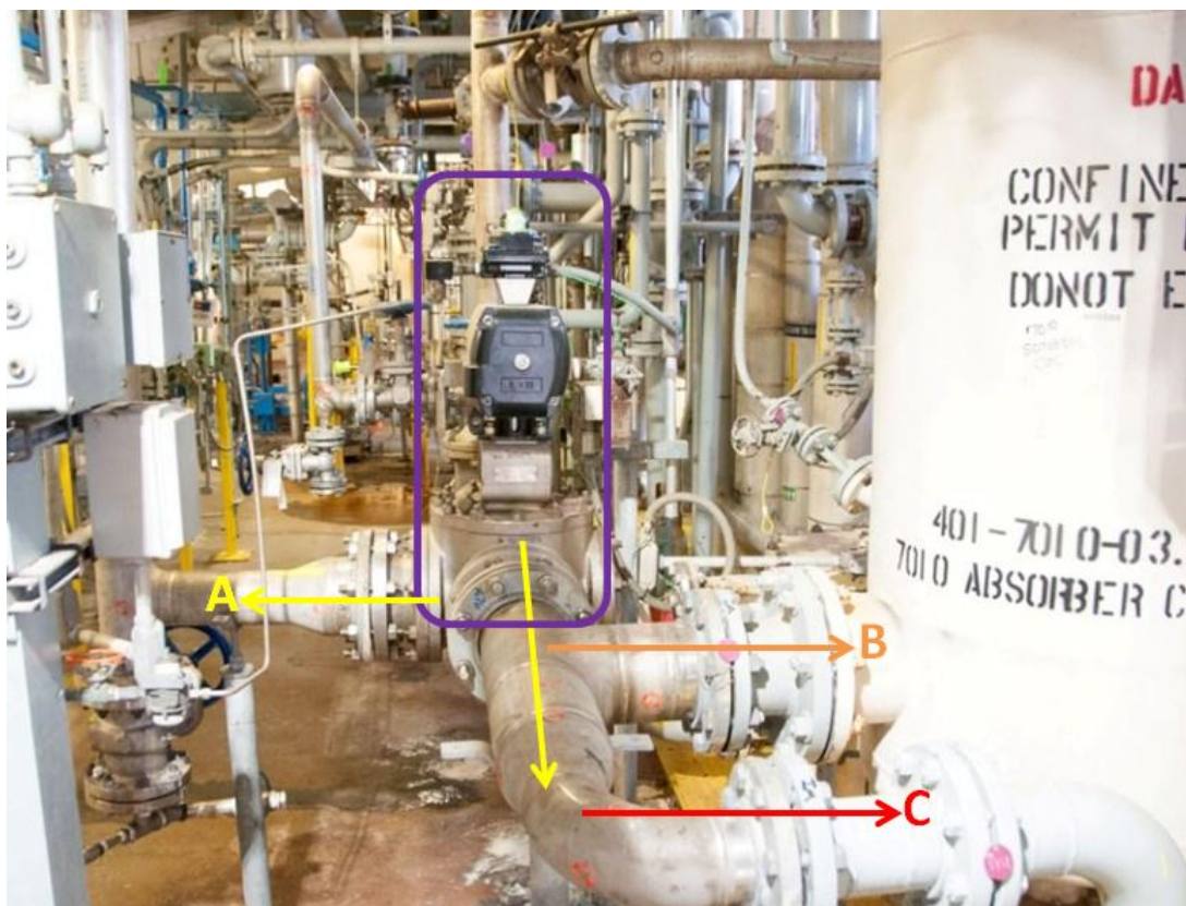
Figure 11. Waste gas vent header piping on the 3 rd floor of the manufacturing building. This photograph was taken while facing north. Figure 10 shows the same waste gas vent header piping but taken while facing south. A 3-way valve (purple) is controlled to send the waste gas to either the NRS incinerator labeled “A” (yellow) or a caustic scrubber labeled “B” (orange). The caustic scrubber is designed with a vapor equalization line labeled “C” (red) that connects to the vapor space of the caustic receiver on the floor below (2 nd floor). Prior to the installation of the NRS Incinerator, the 3-way valve did not exist and liquid that might accumulate in the waste gas vent header piping could freely drain into the caustic scrubber system.
