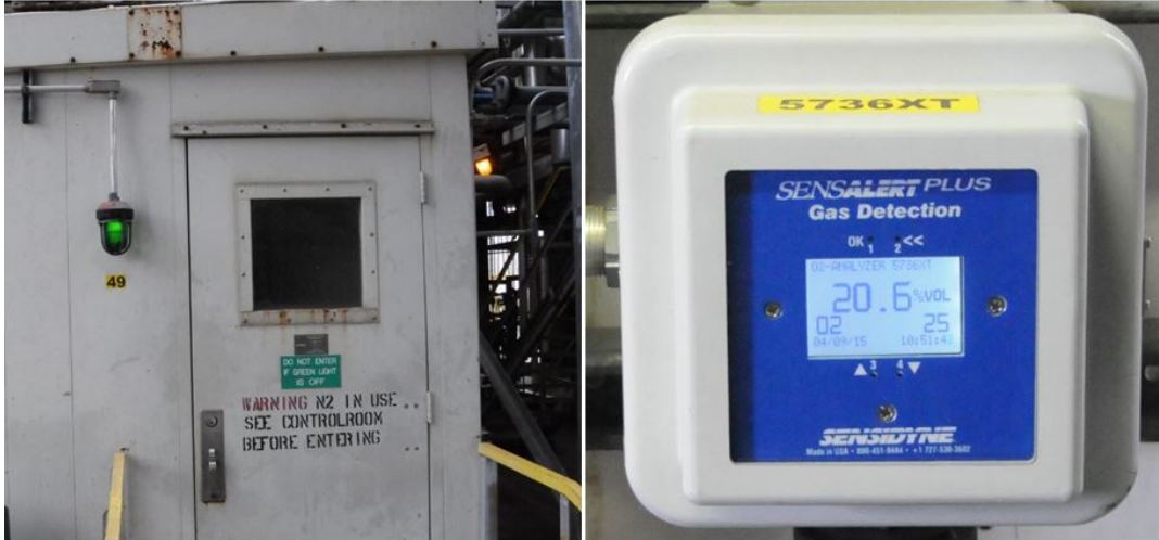
Figure 23. Unlike the manufacturing building this DuPont analyzer house shown in the left photo is equipped with safeguards to ensure entrant safety. The oxygen analyzer shown in the right photo is inside the analyzer house continuously monitoring the analyzer house atmosphere. If a nitrogen leak occurs inside the analyzer house sufficient enough to cause the atmosphere inside to approach dangerous levels, an alarm sounds and the green light outside the door turns off to indicate it is not safe to enter. The manufacturing building lacks similar safeguards. The CSB has not been able to determine why DuPont applied more rigorous safeguards to the infrequently entered analyzer house than for the normally occupied manufacturing building.
