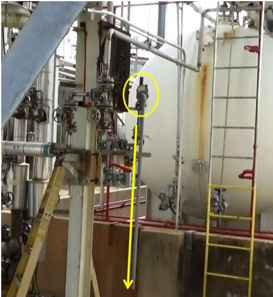
Figure 29. Liquid methyl mercaptan relief valve on the discharge of the methyl mercaptan pumps is designed to discharge this highly toxic, highly flammable chemical to grade just north of the methyl mercaptan storage tank.
