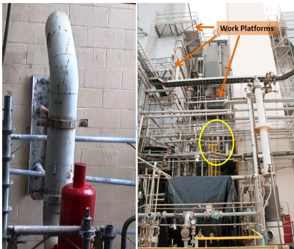
Figure 28. Caustic scrubber pressure relief device location. The photo on the left shows the relief valve within the yellow circle in the photo on the right. This caustic scrubber relief valve is located in a congested area on the north side of the manufacturing building. Although DuPont documentation indicates the discharge piping of this relief valve is 10 feet above the work platform, the analysis failed to consider the other work platforms above this relief valve that can clearly be seen (orange arrows) in the photo on the right. On December 16, 2014, this relief valve was the source of a highly toxic chlorine release when a DuPont operations activity vented chlorine to the caustic scrubber in order to disconnect and relocate a chlorine railcar.
