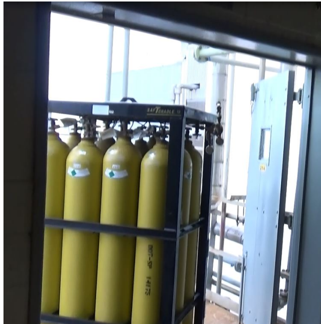
Figure 25. Photo of the open door on the south side of the second floor adversely impacting the dilution air ventilation flow across process equipment described in Figure 24.
