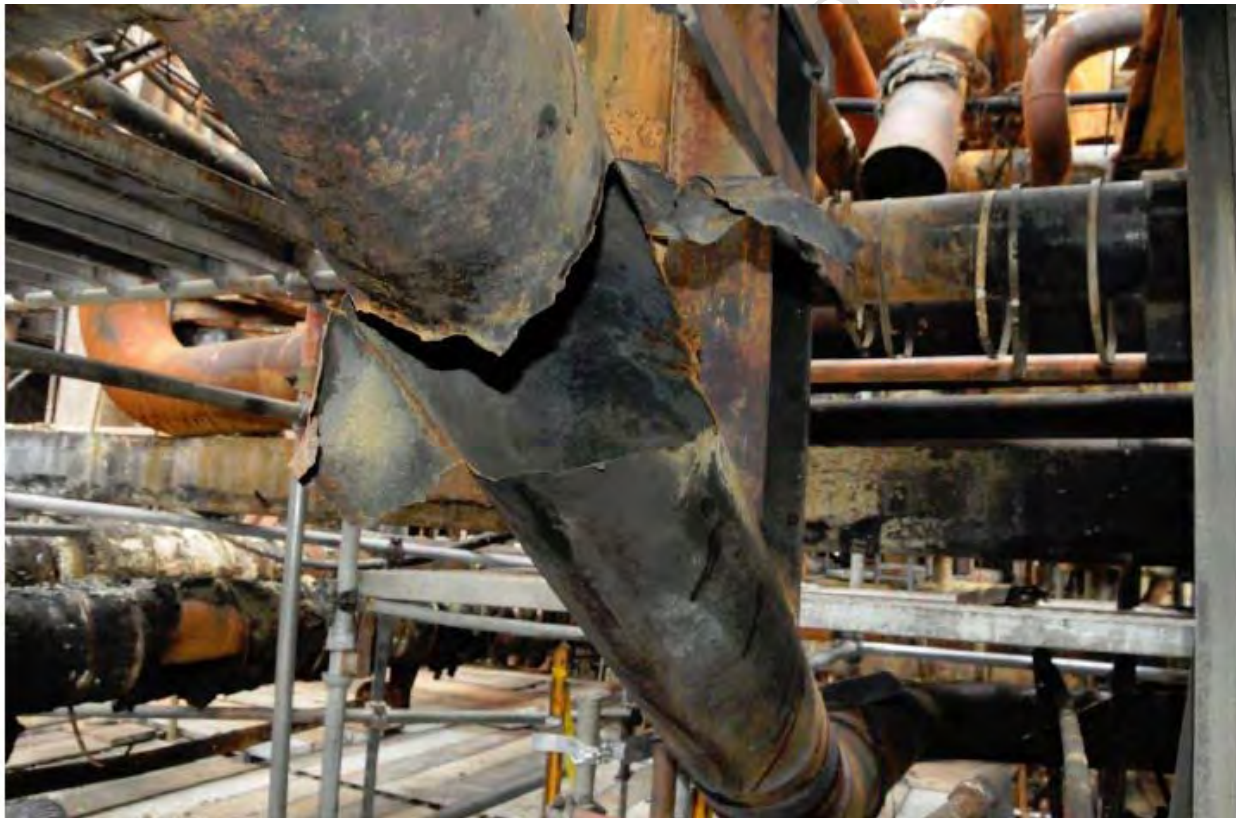
Figure 7. Photo of rupture on 4-sidecut 52-inch component
