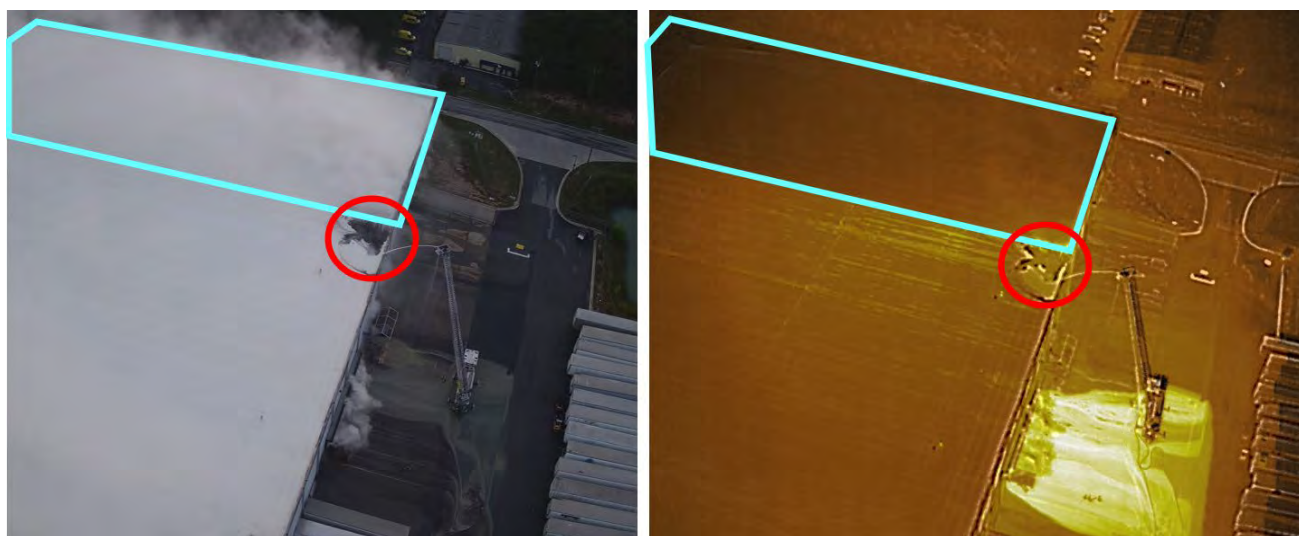
Figure 19. Two images showing the roof membrane damage at 8:11 a.m. after the first was extinguished, with the bunker outlined in aqua and the roof damage circled in red. (Credit: RCFR, annotated by CSB) a
