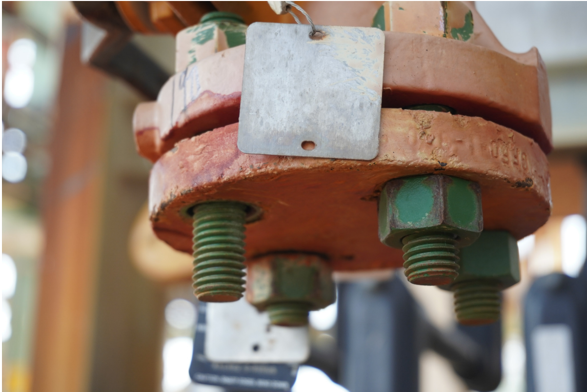
Figure 30. Blind flange as found after the incident. a One nut was removed (foreground left) and another (background left) was loosened to within two to three threads. (Credit: CSB)
