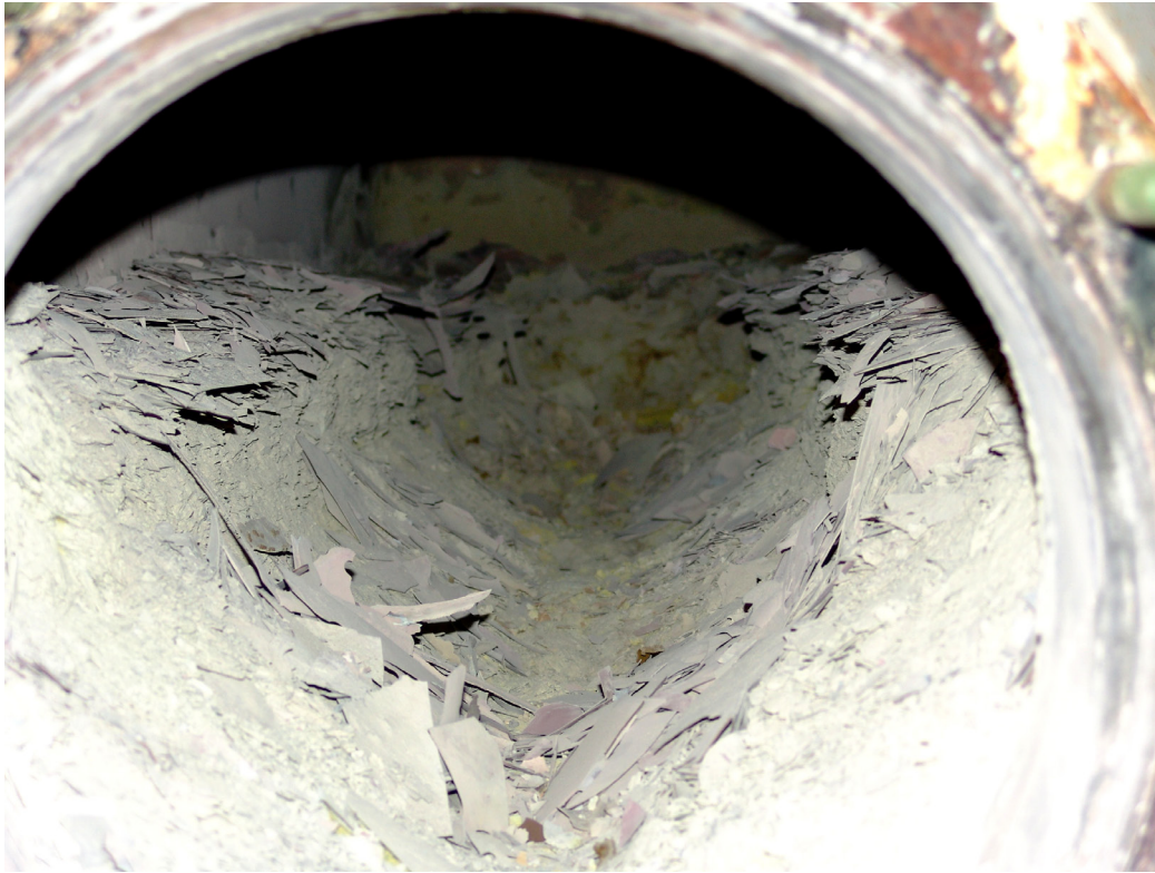
Figure 19. Picture of the inside of the reboiler shell, taken during a May 2005 internal inspection. (Credit: Honeywell)
