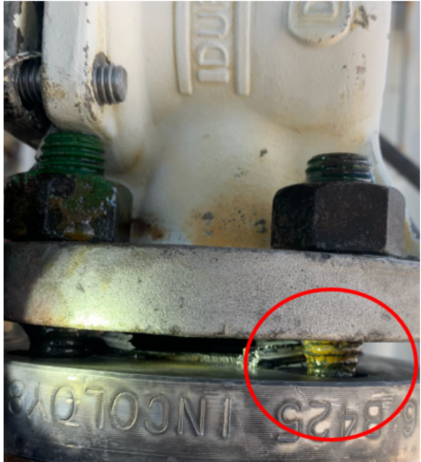
Figure 7. Photo of the flange assembly as found after the incident, showing the stud corrosion observed by the field operators prior to the release. (Credit: Honeywell, annotated by CSB)
