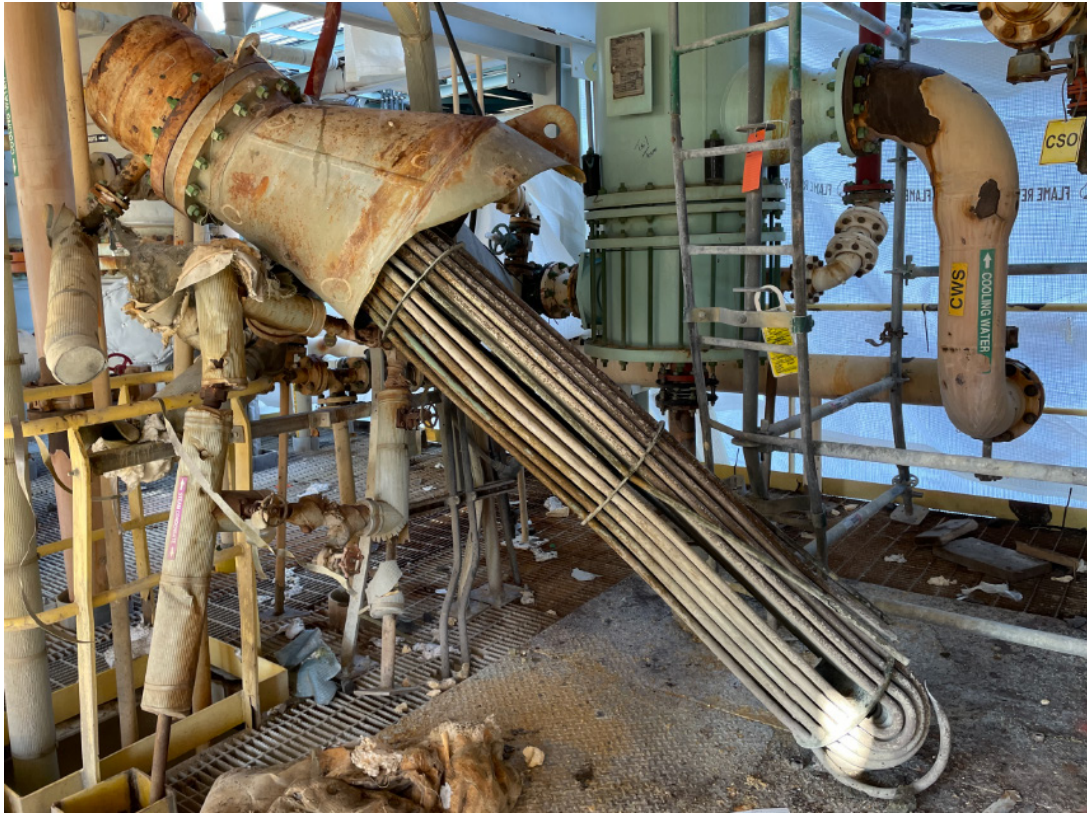
Figure 18. Post-incident image showing the remnants of the reboiler. (Credit: Honeywell)
