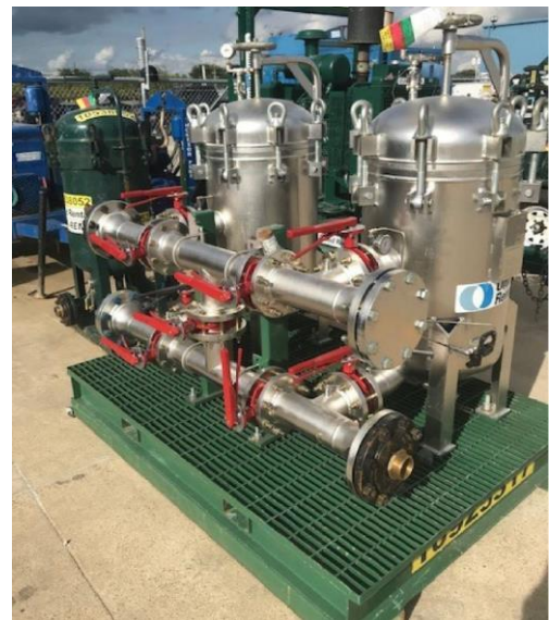
Figure 35. Temporary filter skid – exemplar. (Credit: TPC)
